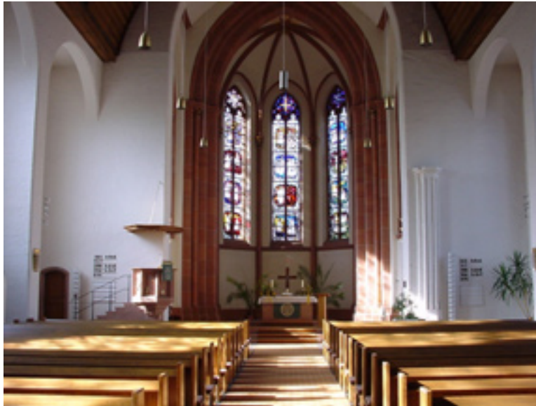
Figure 21. The custom designed line arrays blend in nicely next to the altar.
